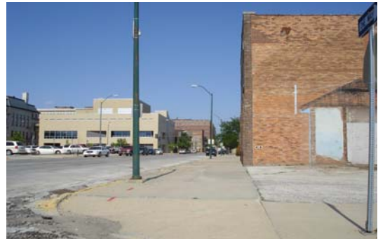
There are several sidewalks and ramps that need maintenance and concrete work within the study area.
