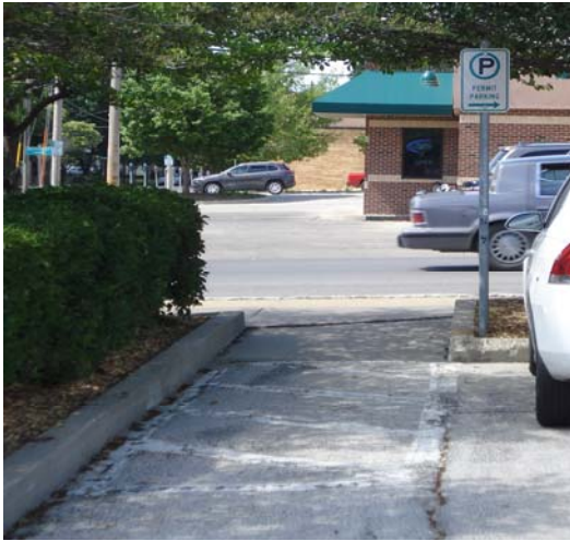
This is an example of a clearly defined walkway within a parking lot in lot #11. The striping should be maintained on an annual basis.
