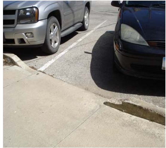
This walkway in lot #12 is ramped, though a vehicle can park on the walkway defeating the purpose.
